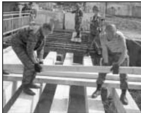
BRIDGE—Two Russian soldiers (above) place decking on bridge spans during a bridge re-construction in the town of Janja, while Staff Sgt. Steven McMinn, 648th Engineer Battalion (below) lowers a beam in place over the bridge.
