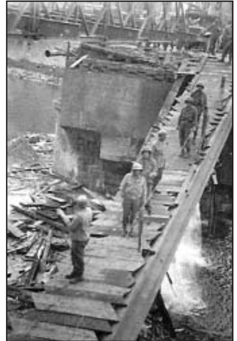
A&P Platoon of the 2nd Bn 30th, made a makeshift foot bridge.
